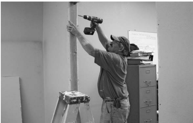
Carpenter Phil Mosconi conducts office renovation at YOTO courtesy of NCH Corporation.
